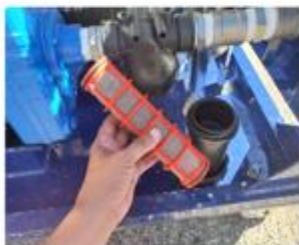
Check and Clean Strainer If Necessary
